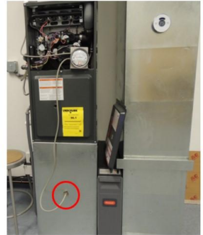
Static Pressure tap at inlet
